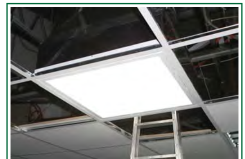
Step 12 - The finished result should look like this. You can now put the surrounding ceiling panels back in place.
